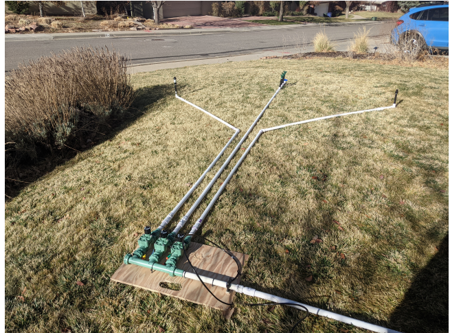
Fig. 15. Custom made Sprinkler Array
