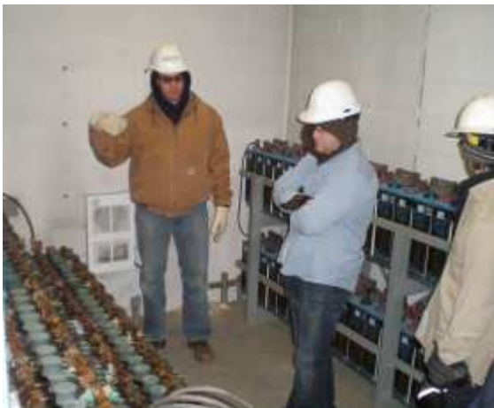
The battery room at Terminal substation (Am)
