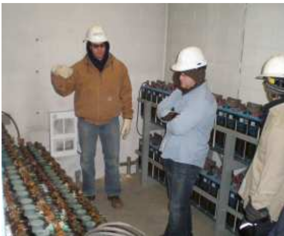
The battery room at Terminal substation (Arn)
