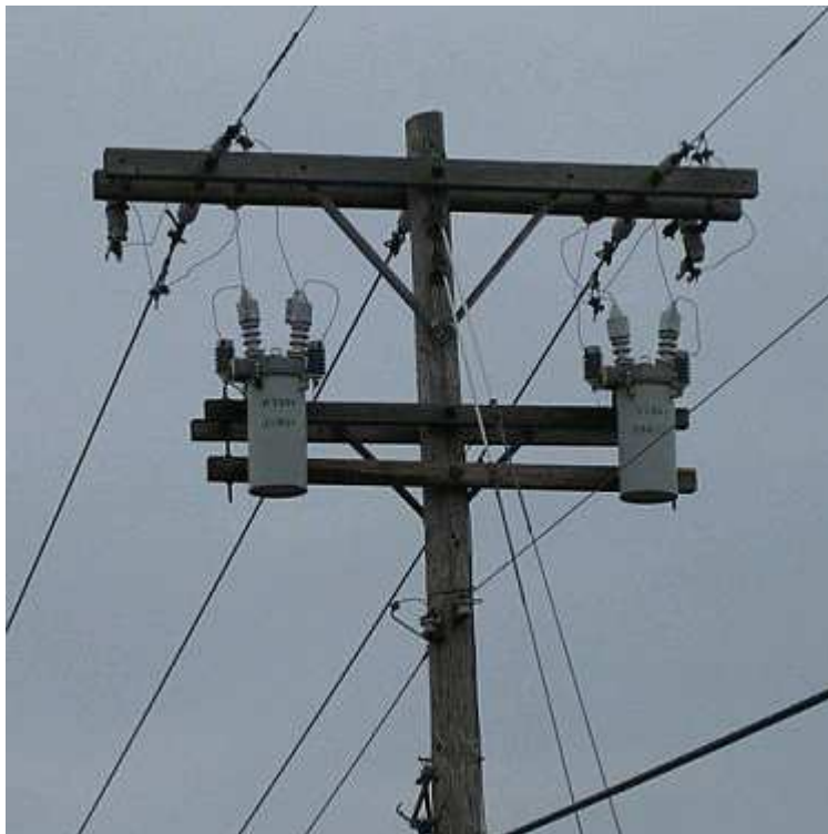
Pole-mounted Reclosure Devices (Eaton)
