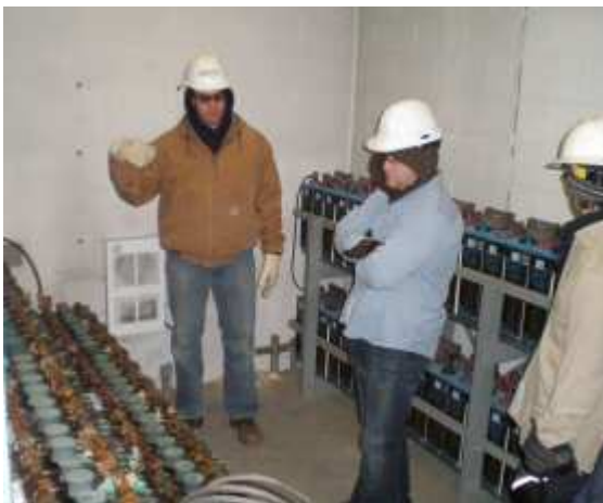
The battery room at Terminal substation (Am)
