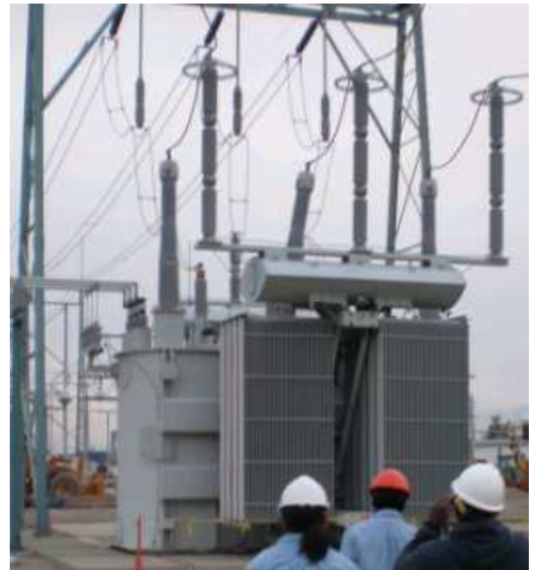
345kV/138kV Autotransformer at Terminal Substation in Salt Lake City. Note oil tank and cooling fins. (Am)
