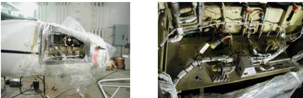
Figure 3. Forward avionics compartment and location of on-aircraft wiring diagnostics test bed.
