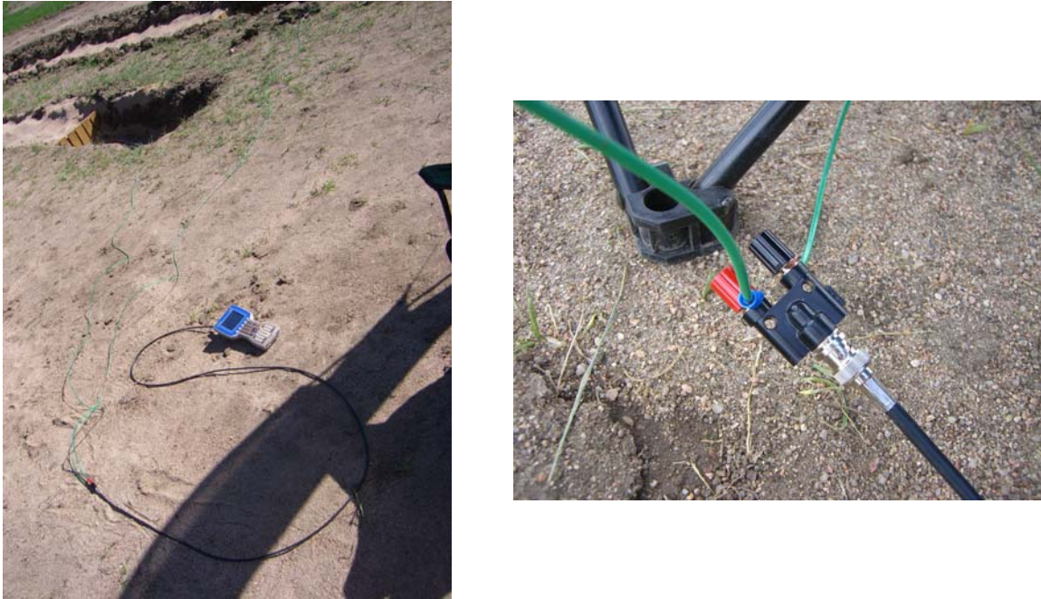
Figure 14 Connection of DATU to simulated anchors in trenches 3 and 4. Care was taken to minimize the coils or loops in the 12 gauge (green) connection wires. (Left photo) 12 gauge wires were connected to the 90 ohm coaxial cable using a banana-to-BNC connector as shown in the right photo. Testing on subsequent days was made easier (on our fingers!) by soldering banana plugs to the 12 gauge wires, so they could be simply plugged into the banana jacks.
