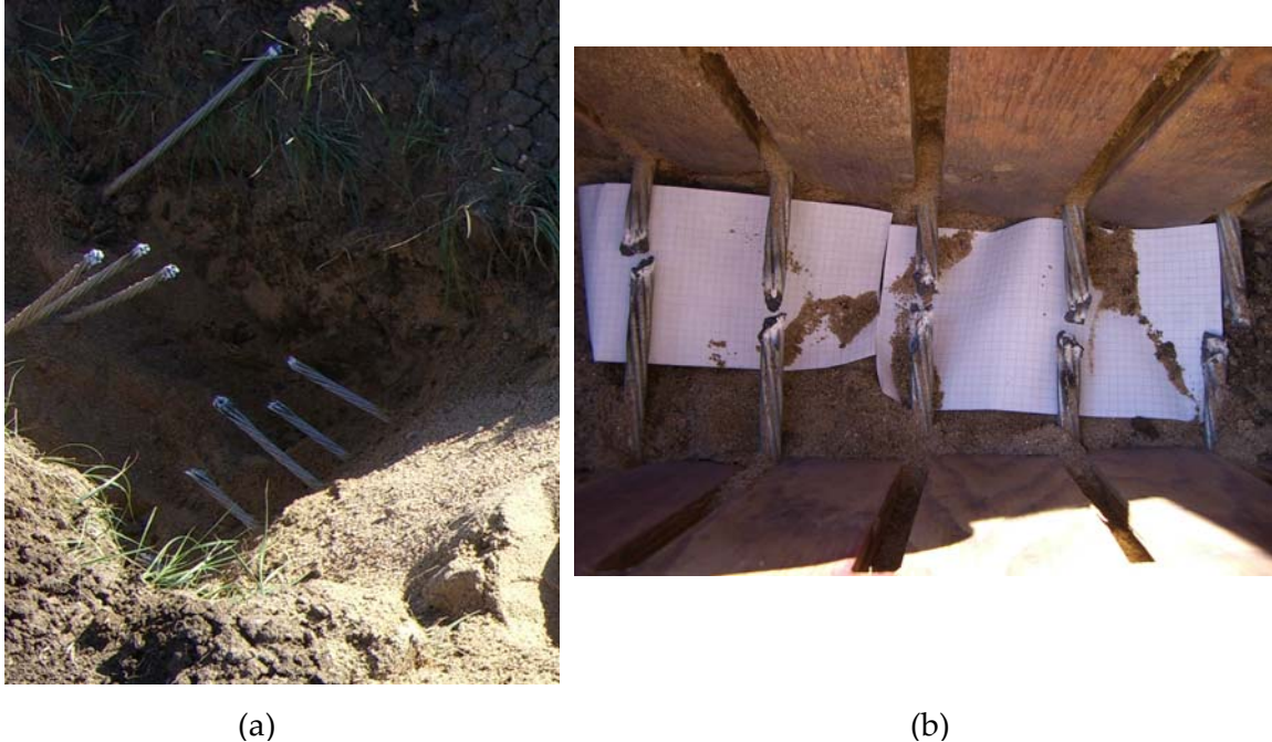
Figure 15 Simulated Damage. (a) shows five strands completely cut and pulled away from each other. (b) shows strands that were cut and not pulled away from each other. Both fault types gave similar results.
