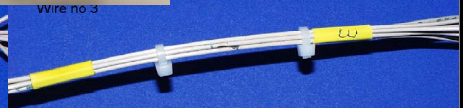
AFCI Tripped on "Wet Arc"
